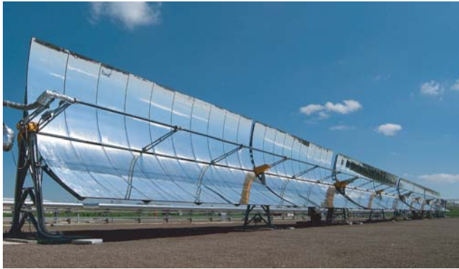
PCS system for solar components (ENEA Casaccia Research Centre)
